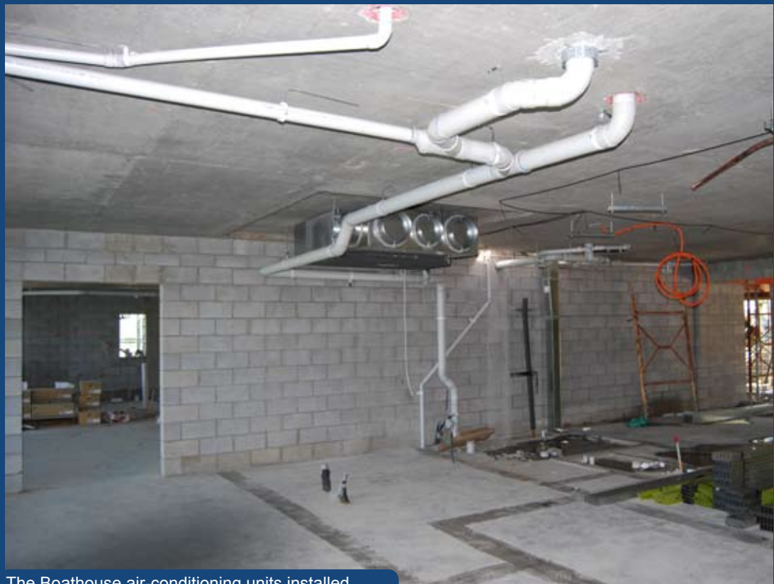
The Boathouse air-conditioning units installed
